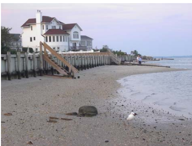
Photos 30 to 32. Shore protection structures can block the inland migration of mudflats, vegetated wetlands, and estuarine beaches. Top: a retaining wall along tidal flats in Westchester County, New York (March 2003). Middle: a bulkhead along a tidal marsh in Monmouth, New Jersey (September 2003). Bottom: a bulkhead along South Jamesport Beach in Riverhead, New York (September 2006). Photo source: ©James G. Titus, used by permission.
