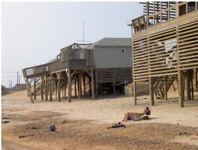
Photo 9. Exposed septic tank makes beach home uninhabitable. Kitty Hawk, North Carolina (June 2002). Photo source: ©James G. Titus, used by permission.
